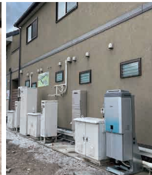
Installed 100% hydrogen combustion water heaters
